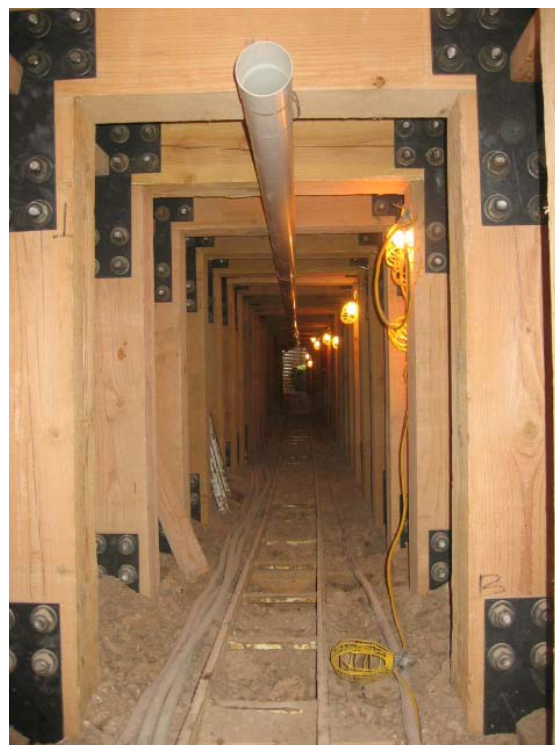
Figure 2. Photograph of the inside of the tunnel displaying the wood shoring, rail tracks, ventilation pipe, and electrical lighting.
